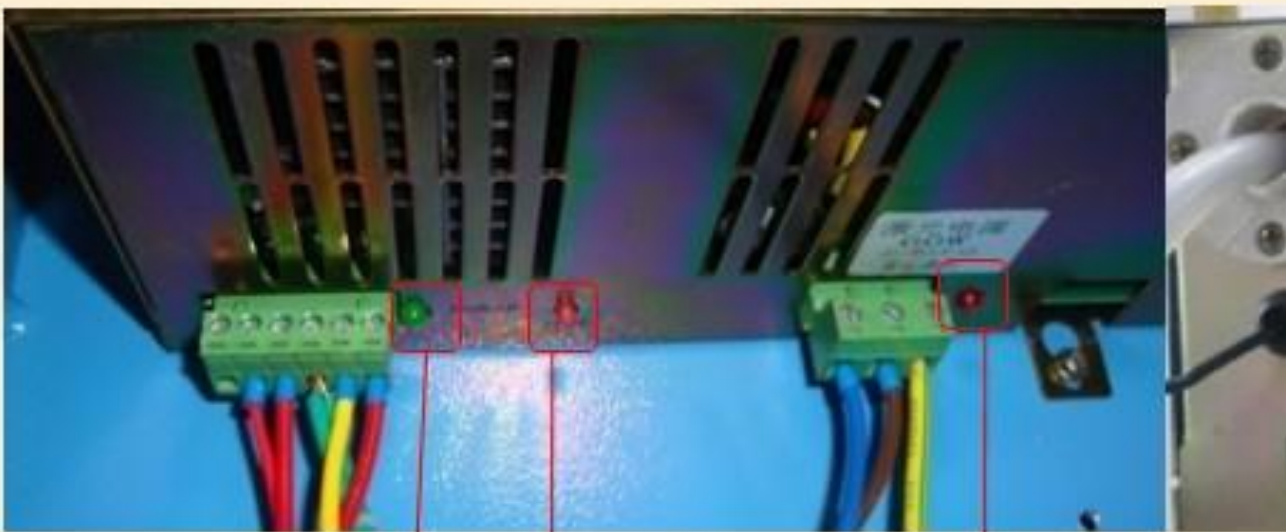
Power indicator lamp
